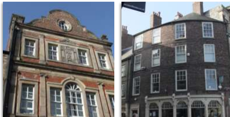
Image 130 Quality of rainwater goods varies
