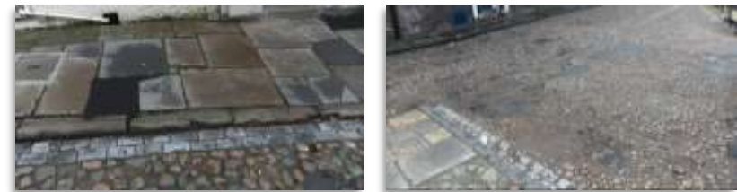
Image 121 Poor repairs to the floorscape
