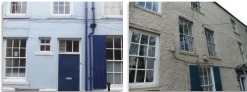
Image 120 maintenance issues and clutter from wiring
