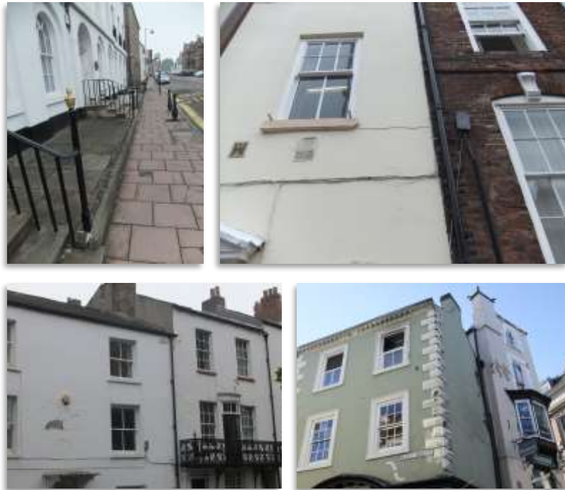
Image 58 Missing railings, cable clutter and examples of peeling paintwork
