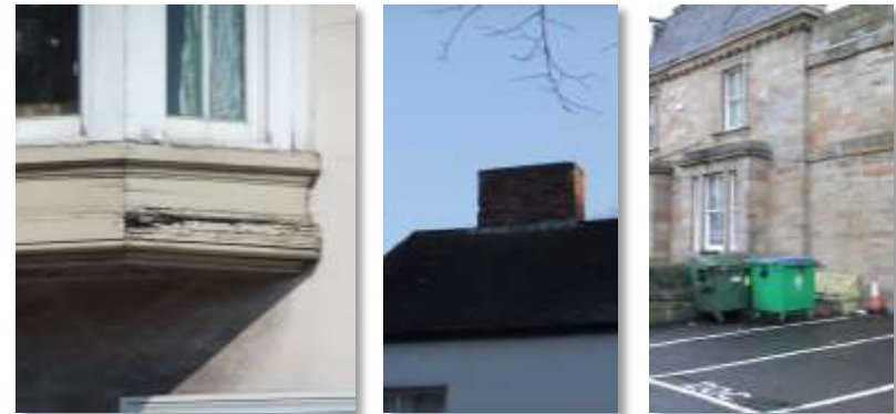
Image 59 Rotten timberwork, missing chimney pots and commercial bins
