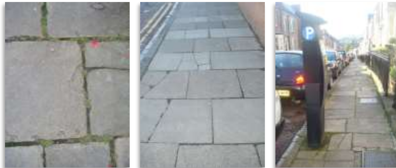
Image 19 Paving is of variable quality
