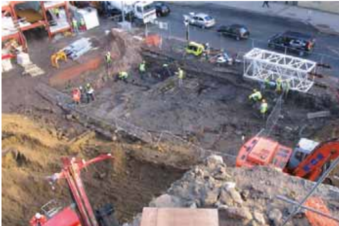
Figure 78 Excavation of post-medieval stone buildings at Tuthill Stairs, Newcastle upon Tyne (Tyne and Wear). ©Tyne and Wear Museum Services
