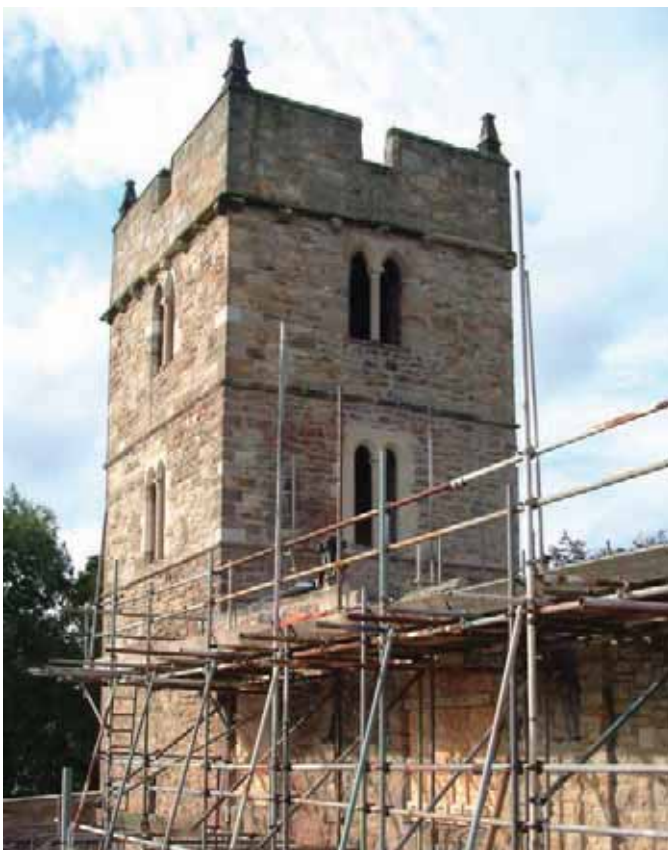
Figure 93 Conservation work on the tower of St Brandon's, Brancepeth (Co. Durham), following the catastrophic fire of 1998. © Peter Ryder
