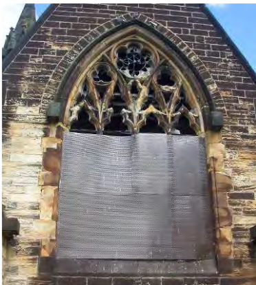
The mortuary chapels are in a particularly poor state of repair
