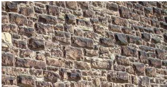
Squared, uncoursed stone work with a slight rockface finish – the most common form of construction in the conservation area.
