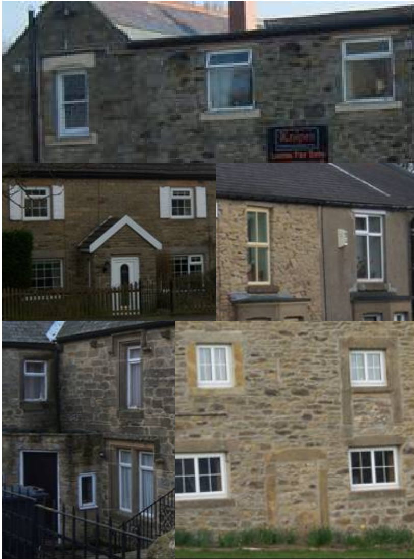
Examples of modern windows in historic buildings. These detract from Edmundbyers' historic character.
