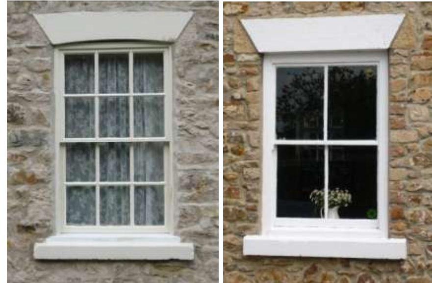
The uncut ends of the lintels were intended to be hidden by render, now removed
