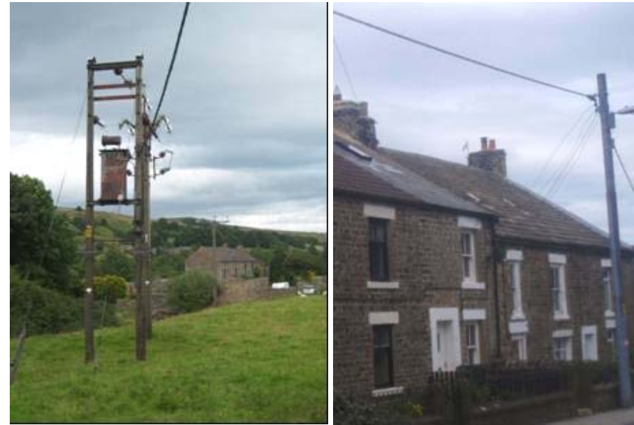
Overhead power infrastructure, poles and lines
