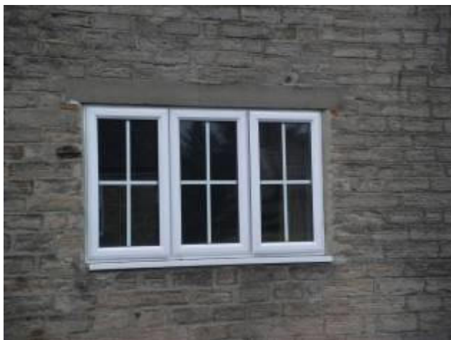
Modern windows of poor quality
