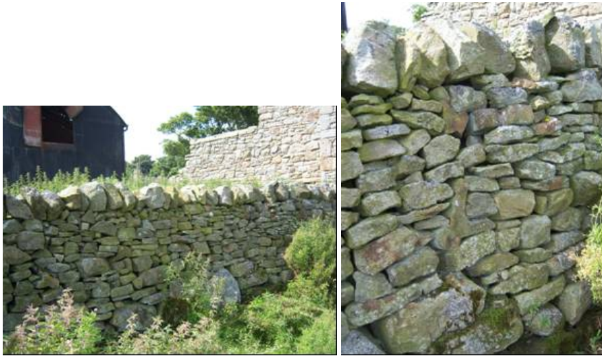
There is a high potential for stone walls at Muggleswick to contain worked stone from the medieval grange. This section of wall adjacent to the Grange ruins contains several ridge stones from the medieval roof.
