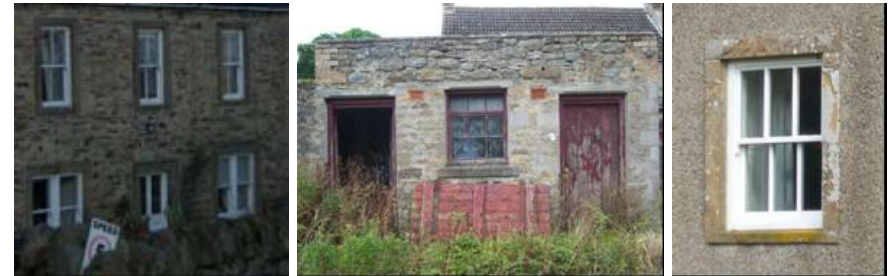
A range of doors and windows of various dates within historic buildings at Muggleswick
