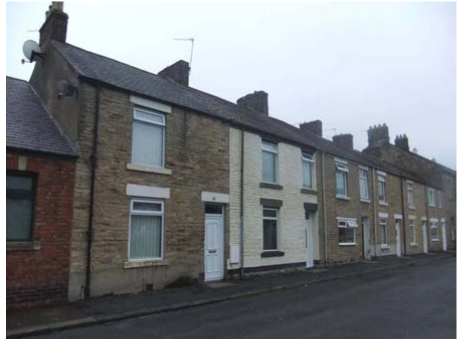
Example of loss of group unity – the terraces on Soho Street have lost much of their character and unity due to poorly replaced windows, window blocking and variations in wall treatment
