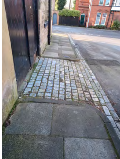
Historic scoria bricks to outbuilding, alongside low-quality concrete paving
