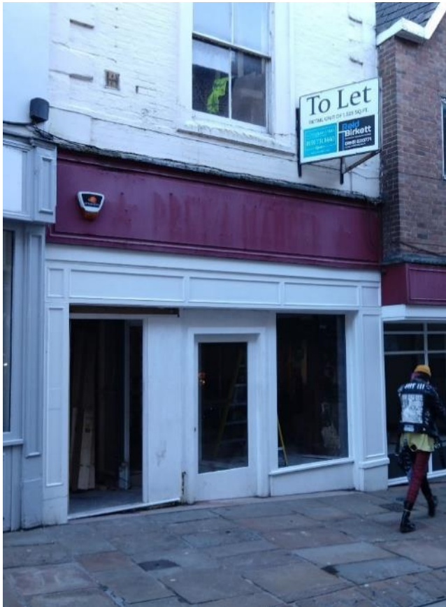
Fig 6 an example of an empty retail unit in Silver Street undergoing refurbishment prior to reuse.
